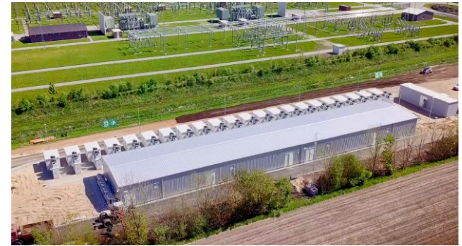
48 MW / 50 MWh, EnspireME, Jardelund, Germany
