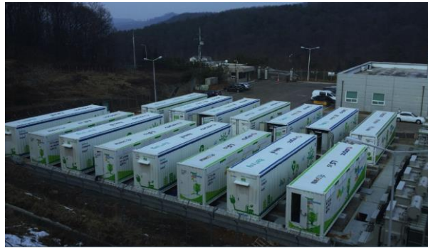
16 MW / 6 MWh, Shin-Chungju Substation, South Korea
